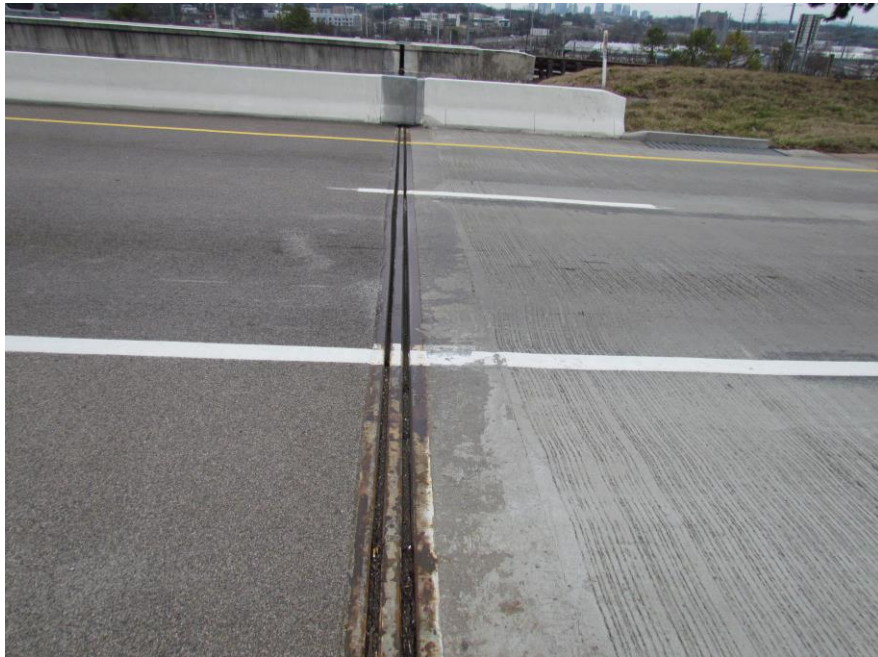
EXPANSION JOINT "B" W/ DEBRIS BLD-UP
