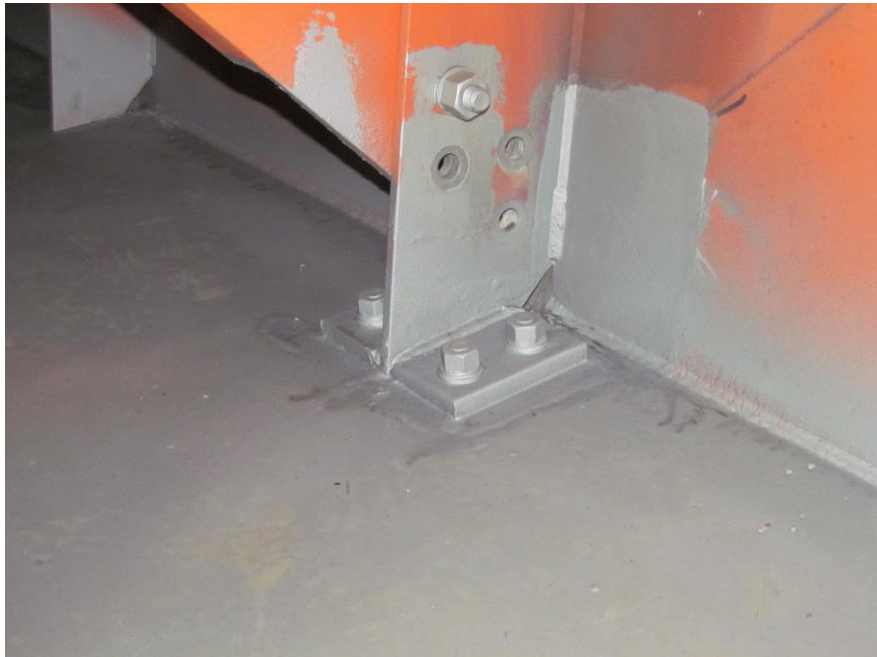
TUB "B" SP. #3 W/ 3 MISSING BOLTS DIAPH. #2
