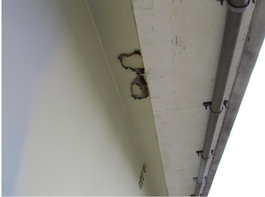
GIRDER W/ PAINT PEELING AT SPAN #6
