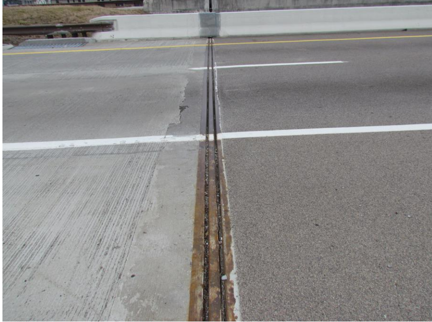
EXPANSION JOINT "A" W/ DEBRIS BLD-UP
