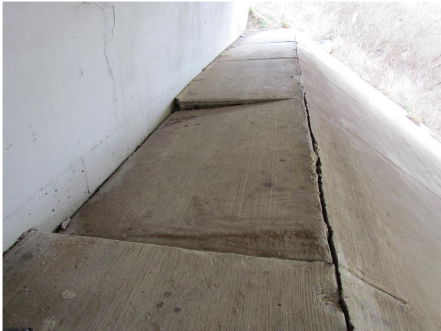
SLOPE PAVEMENT ABUTMENT #2 W/ SAG
