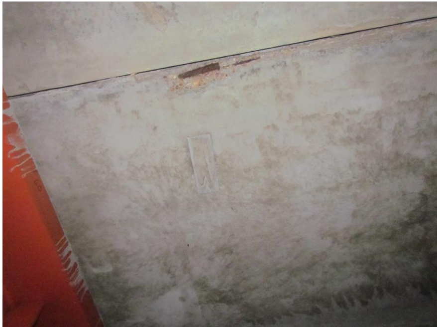
TUB "B" DECK PANEL#1 SP. #3 W/ SPALL & E.S
