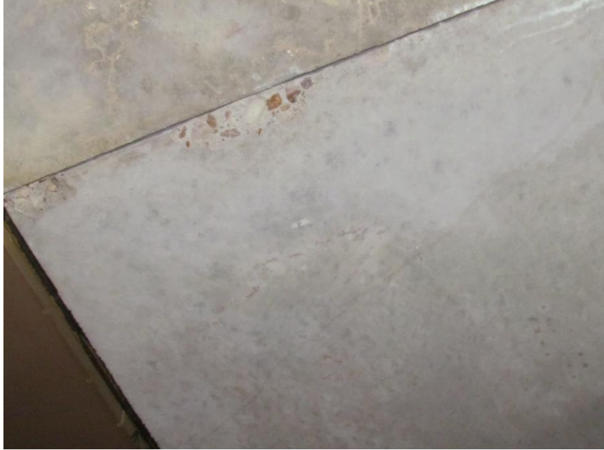
TUB "B" DECK PANEL SP. #4 W/ SPALL
