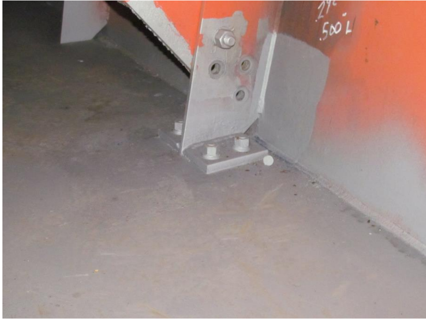
TUB "B" SP.#3 W/ 3 MISSING BOLTS DIAPH. #1
