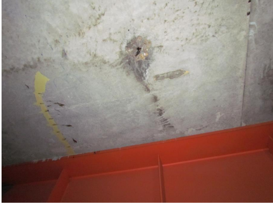
TUB "B" DECK PANEL SP. #3 W/ SPALL
