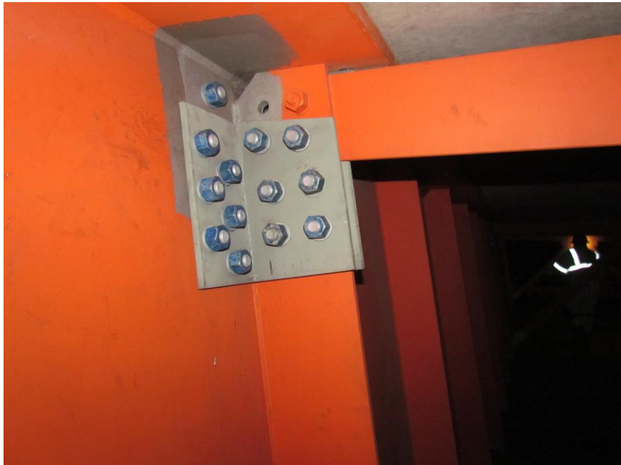
TUB "B" SP. #3 W/ 1 MISSING BOLT DIAPH. #10
