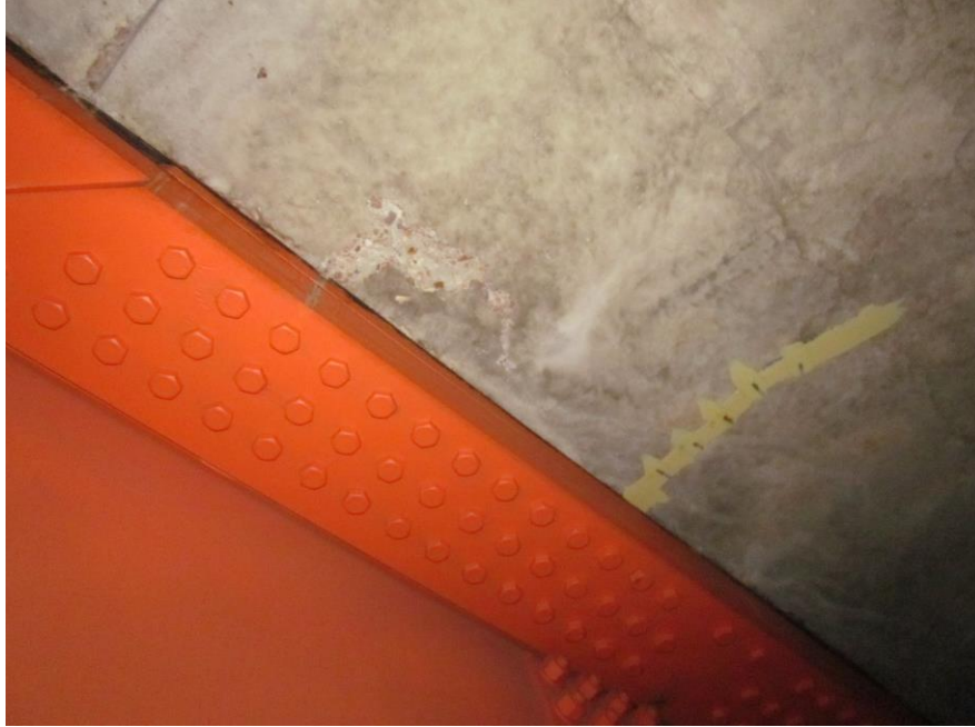
TUB "B" DECK PANEL SP. #3 W/ SPALL
