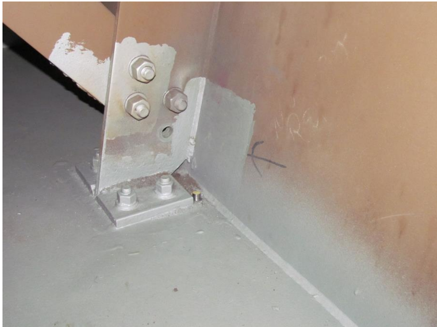
TUB "B" SP. #4 W/ 1 MISSING BOLT DIAPH. #8
