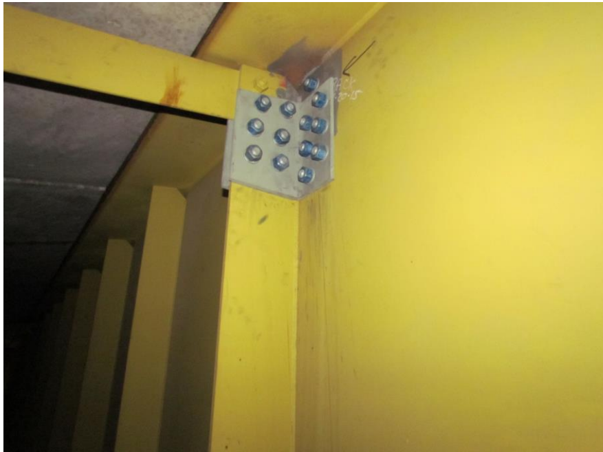
TUB "B" SP. #6 W/ 1 MISSING BOLT DIAPH.#11
