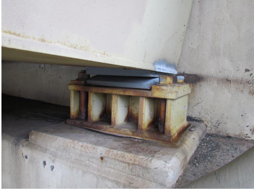
BEARING DEVICE W/ REPAIRS ABUT. #1
