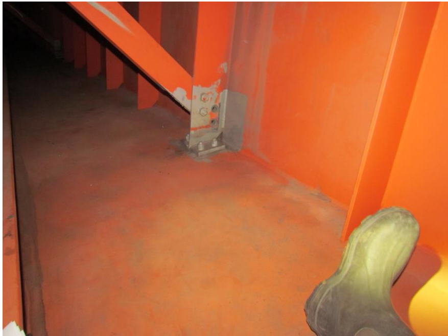
TUB "B" SP. #2 W/ 2 MISSING BOLTS DIAPH.#6
