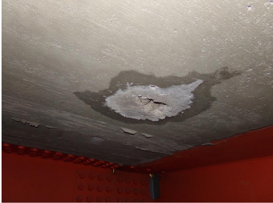
TUB "A" DIAPH.#3 SP.#1 DECK PANEL W/ SPALL
