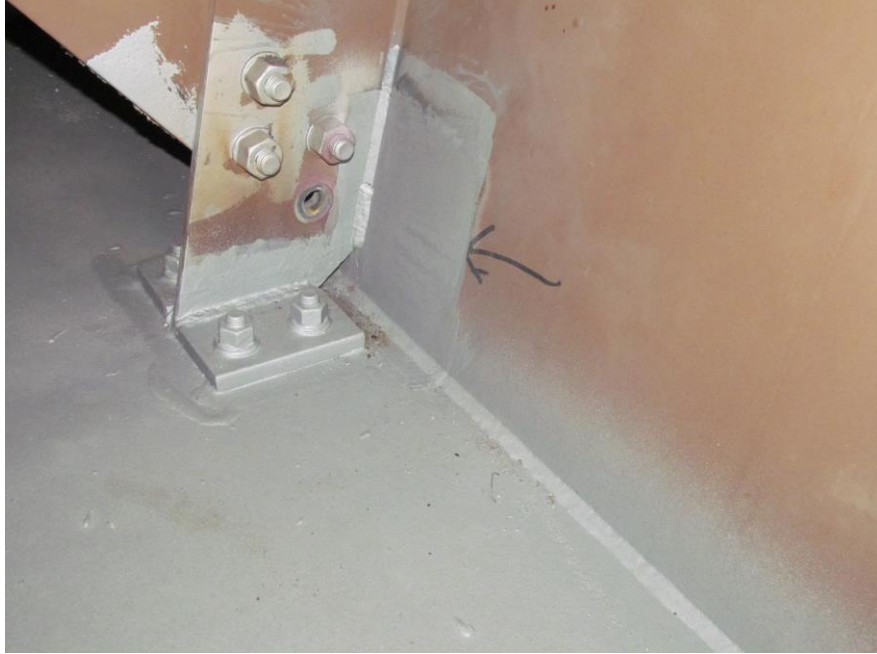
TUB "B" SP. #4 W/ 1 MISSING BOLT DIAPH. #6
